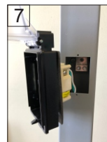
7 Put together the wiring device, gasket, and while-in-use cover and screw to the pedestal post.
