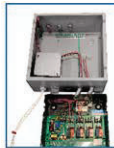
Shown fabricated to lighting panel, used as pull box
