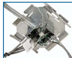
T5B-50/200 shown installed to BCHS-6S in open ceiling, used as a home run box
