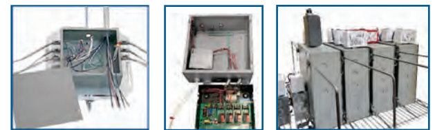
Shown installed to BCHS-12, MC cables connected to 1/2" K.O.'s
